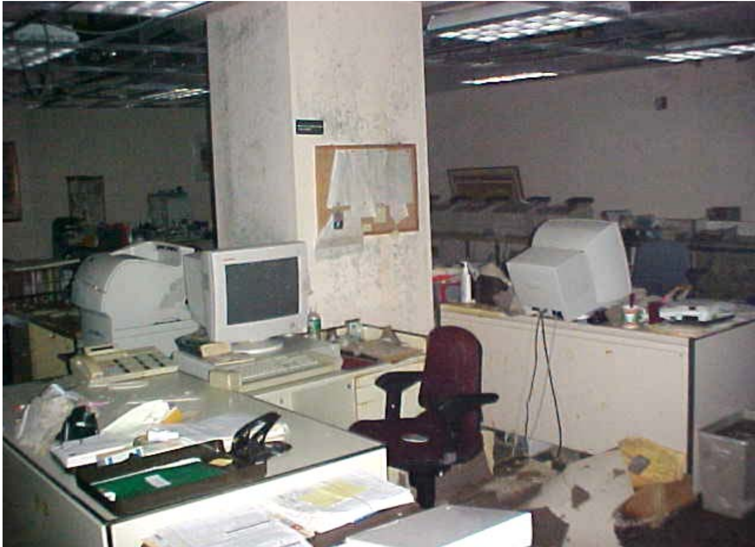
Mold on column and other surfaces - flooded basement
