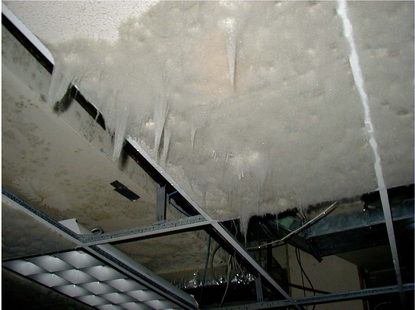
Mold Growth - “woolly” appearance visible
