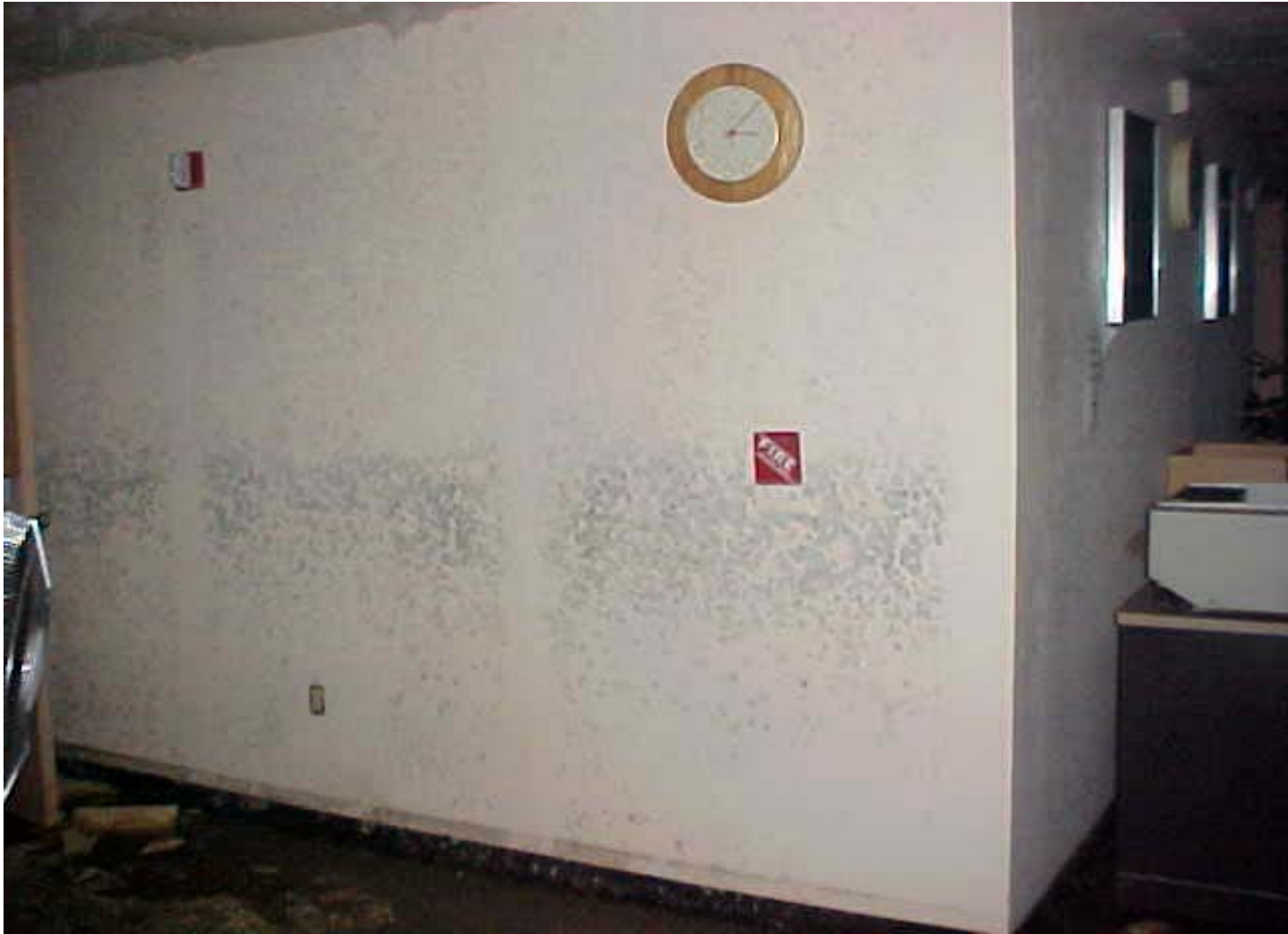
Mold on wall after a flood - 3 weeks of growth
