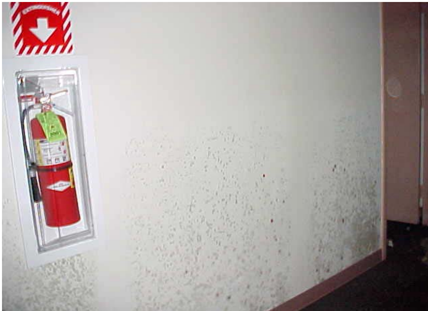
Mold growth on wall board - flooded basement
