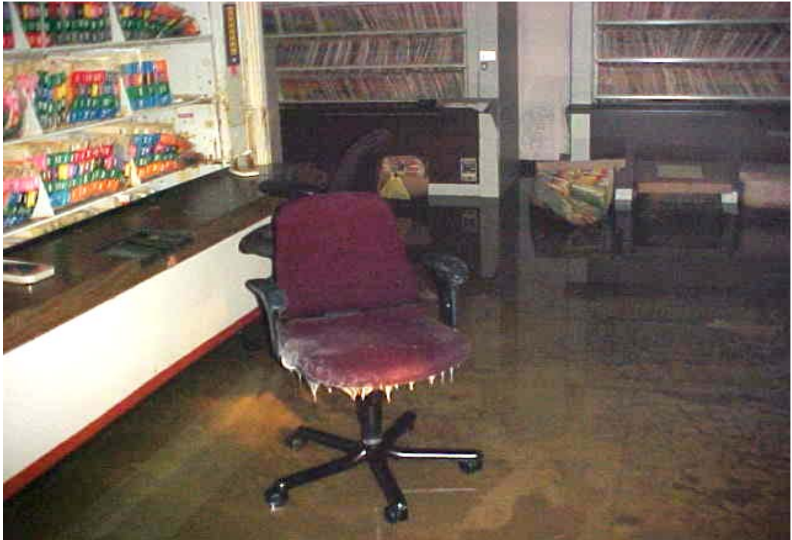
Moldy chair and medical records - basement after a flood
