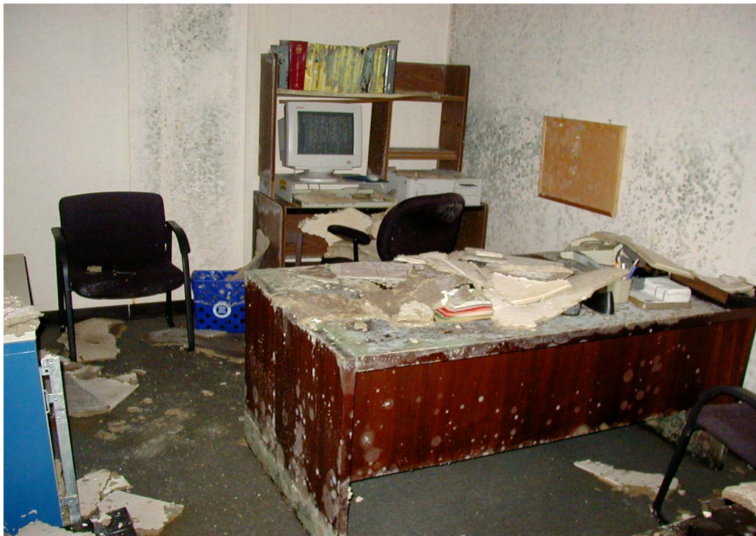
Basement office after flood - 3 weeks mold growth
