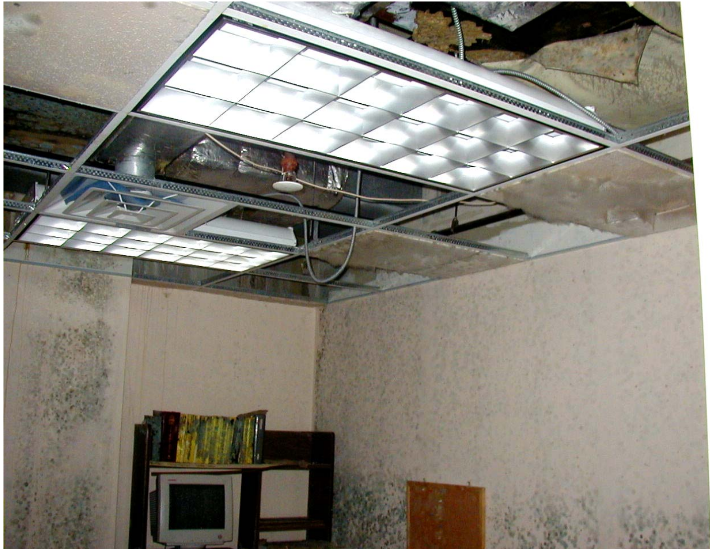
Mold growth on walls and above ceiling - 3 weeks
