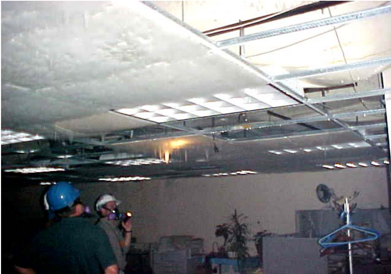
Extreme mold growth in a basement - 6" "fuzz" on ceiling
