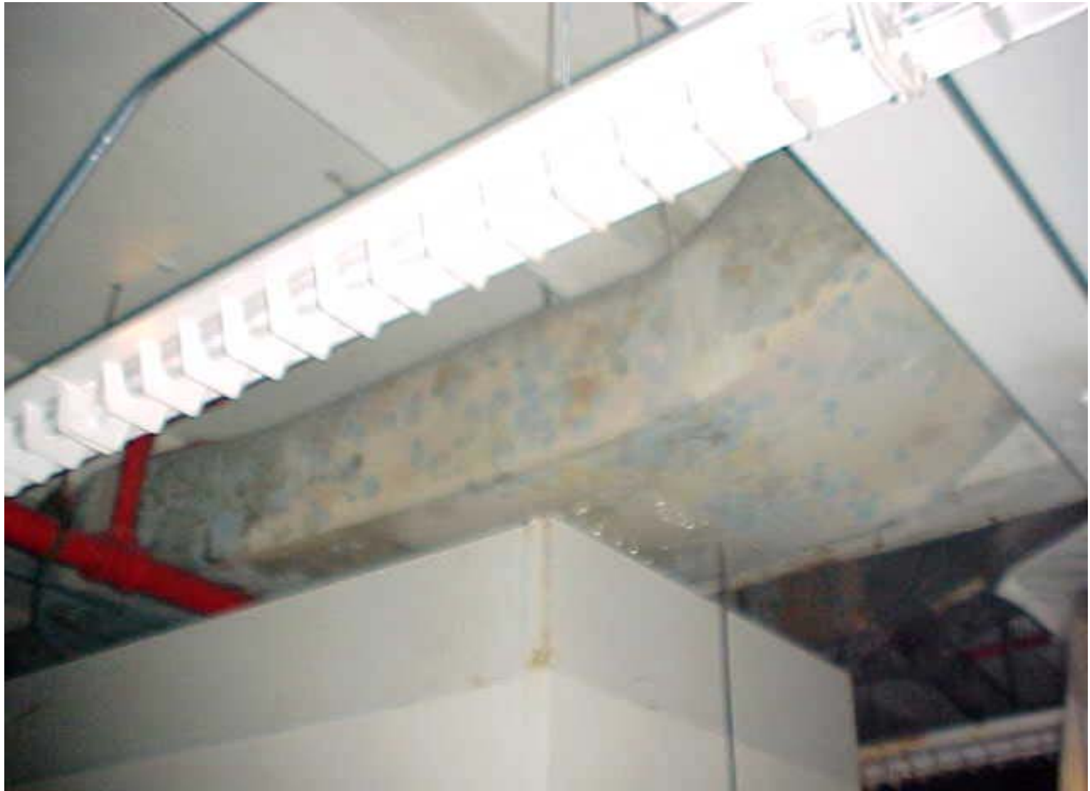
Mold on ventilation duct exterior
