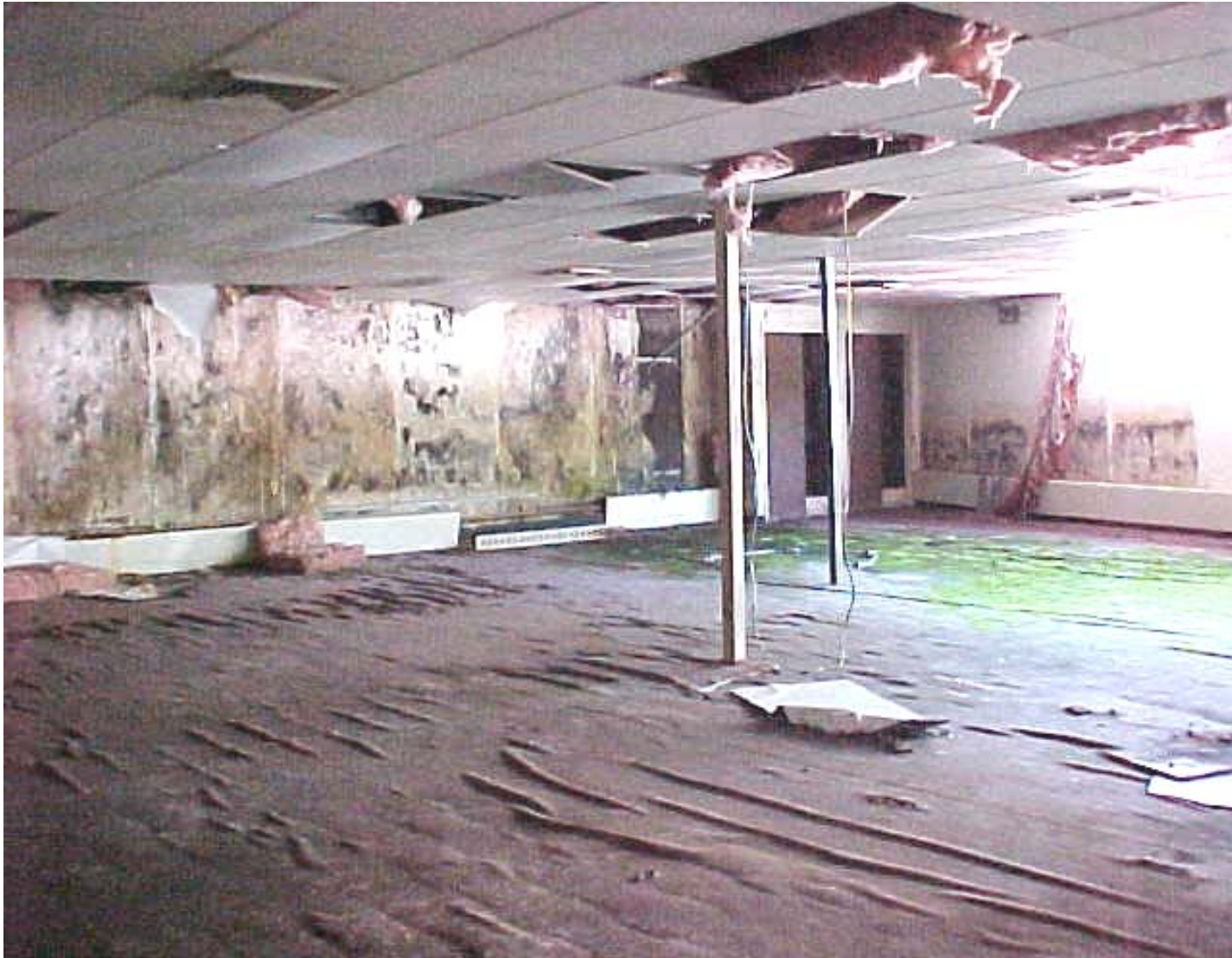
Uncontrolled / Extensive Biological Growth
