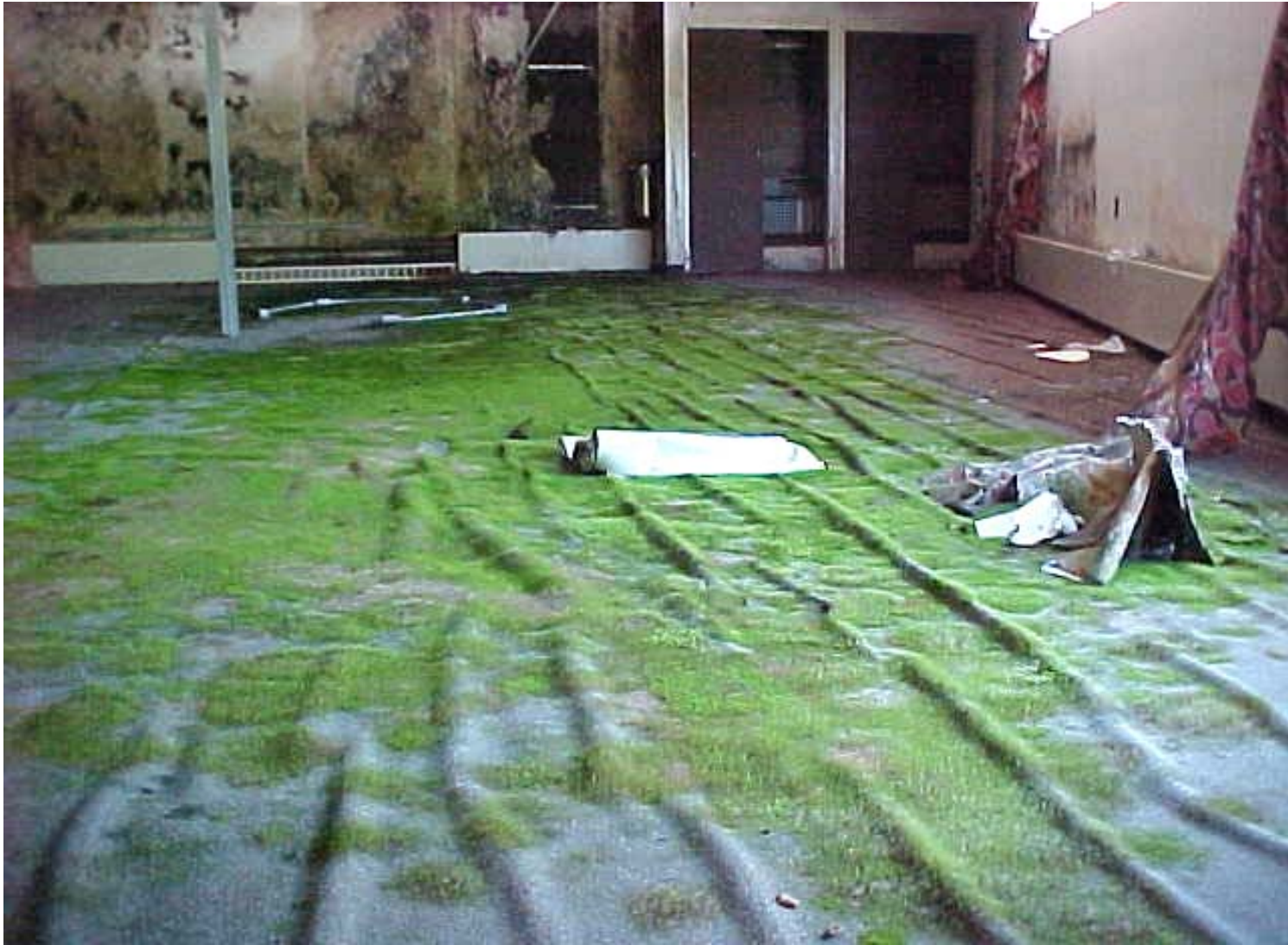
Uncontrolled / Extensive Biological Growth
