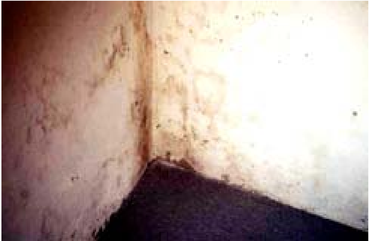
Mold growth in corner of a room (generic photo)
