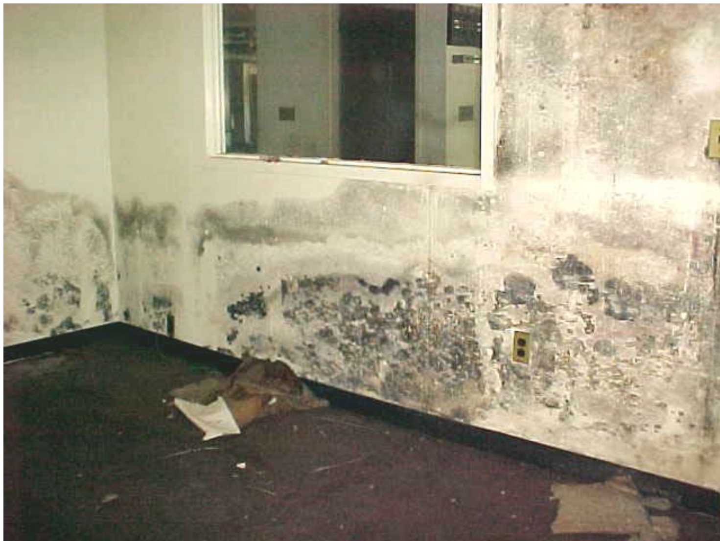
Uncontrolled / Extensive Mold Growth
