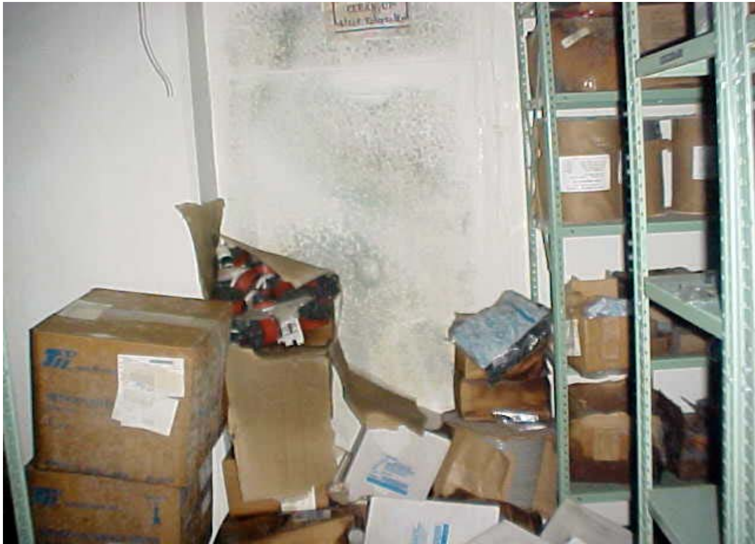
Storage room in basement - 3 weeks of mold growth
