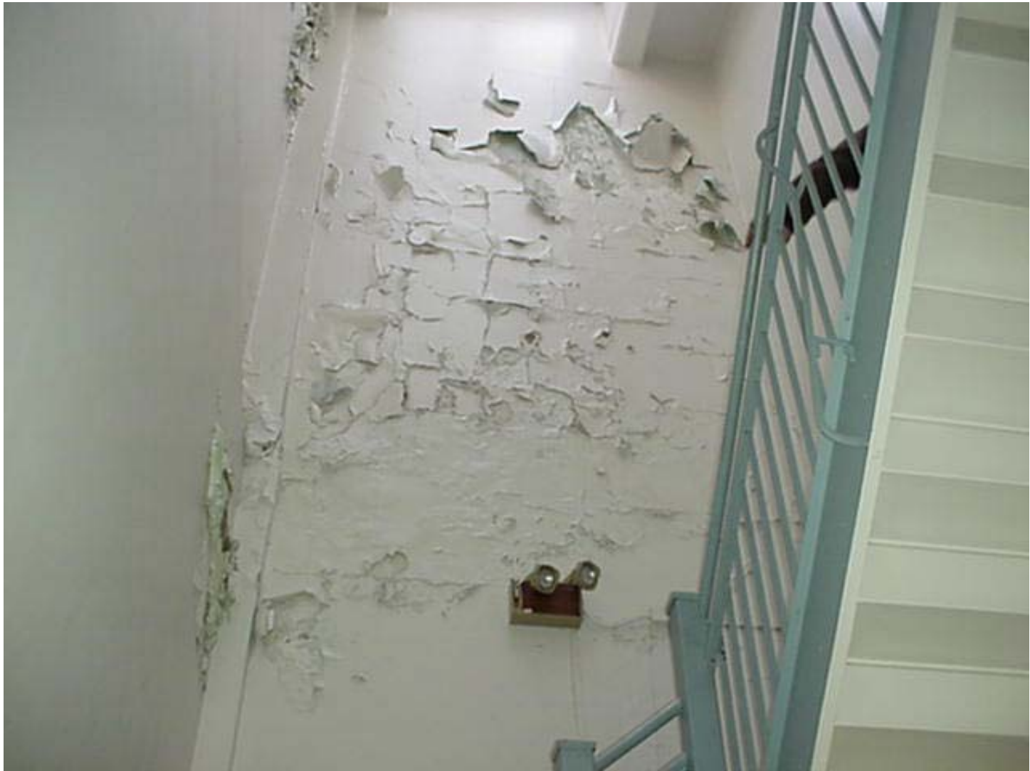
Peeling Paint - Indicative of moisture/water migration
