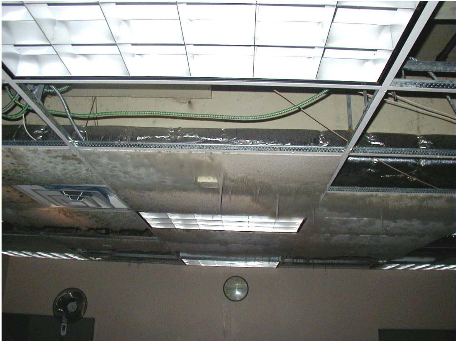
Mold Growth on Ceiling - 3 weeks
