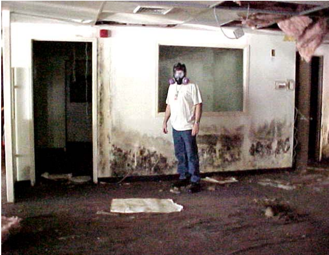
Uncontrolled / Extensive Mold Growth
