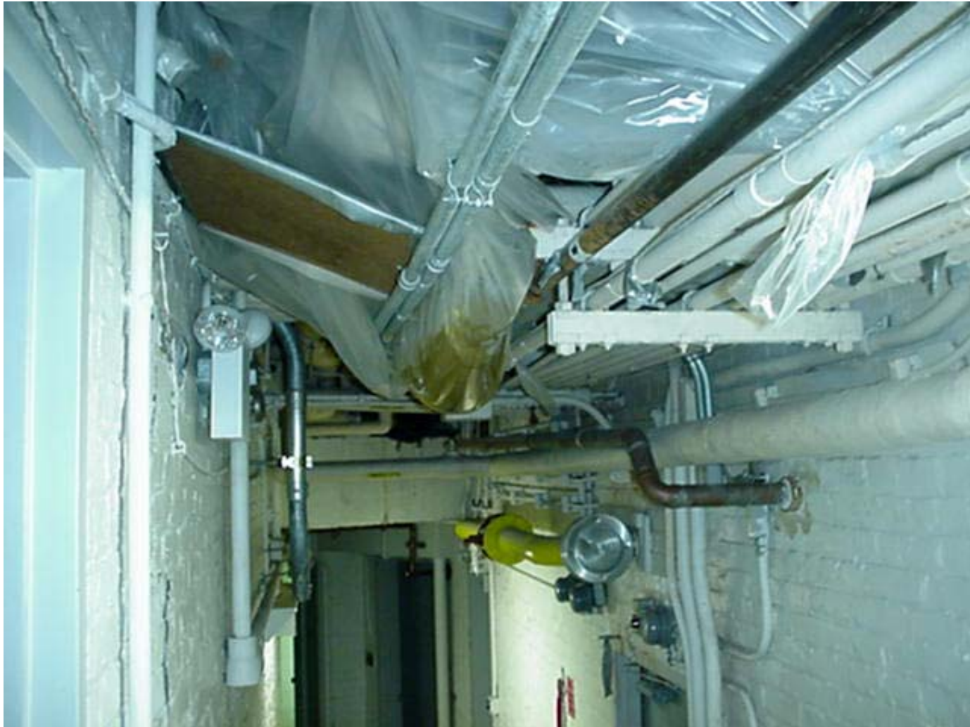
Long-term water leak. Plastic with water accumulation.
